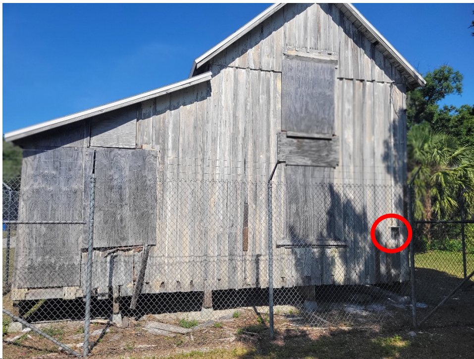
East wall with fuse box (2024)
