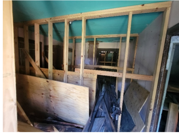
Shoring and Debris at Southeast corner(2024)
