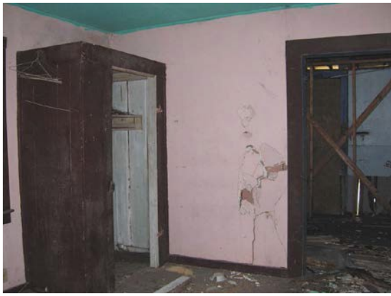
Southeast corner with modern closet. Note the exposed section of vertical board finish on the south side of the wall. (2008)
