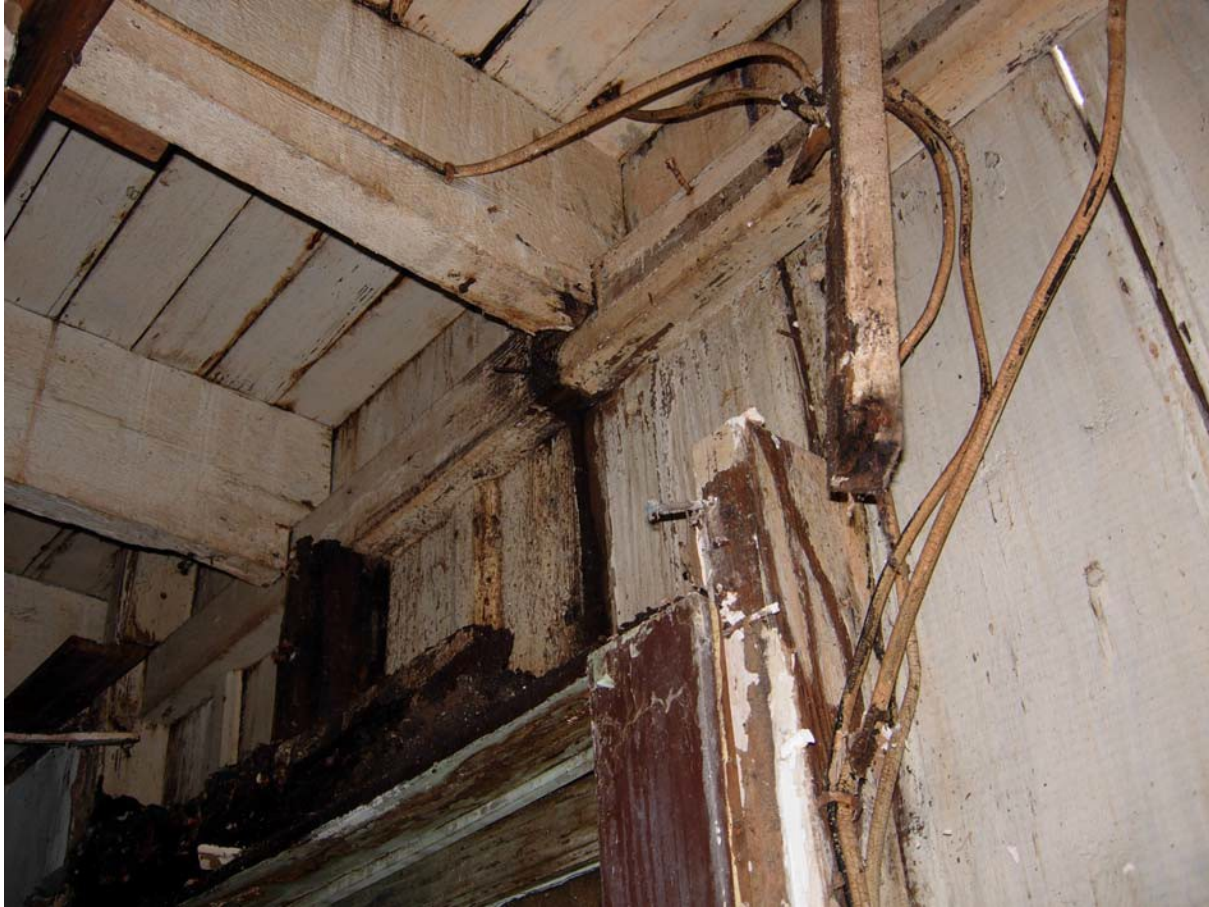
Second floor joists, north wall, notched over ledger which is notched into the studs. Note stud to right of opening was cut off. (2008)
