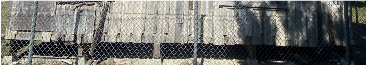
East Side Board and Batten siding severely deteriorated at base of structure (2024)
