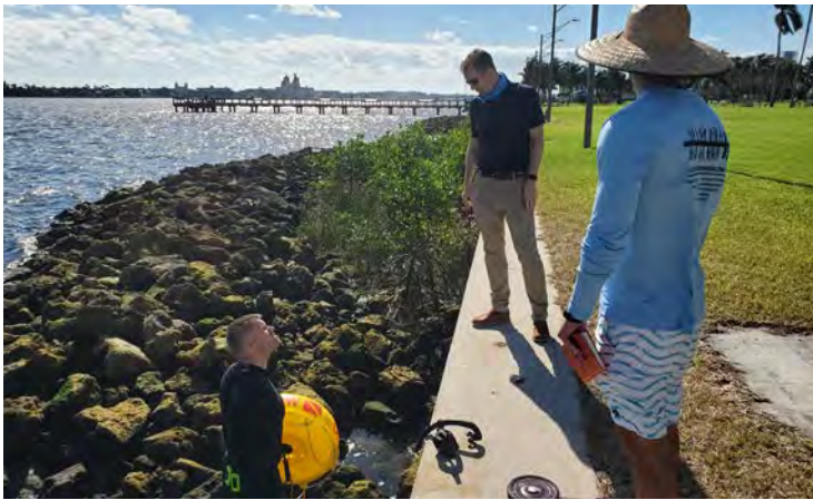
Engineers on site at Currie Park during construction, coordinating waterfront improvements and living shoreline implementation as part of the park's resilient redevelopment
