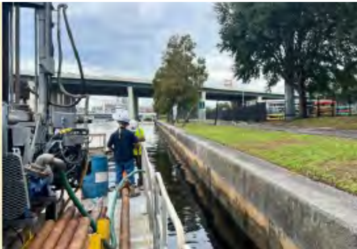
Arehna Engineering provided geotechnical engineering support for the West River Redevelopment and Complete Streets project, contributing to living shoreline and seawall restoration along approximately 12 miles of multimodal infrastructure improvements in Tampa, Florida
