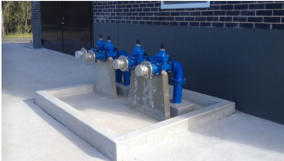
Figure 15 Standpipes exterior to a vacuum sewer station
