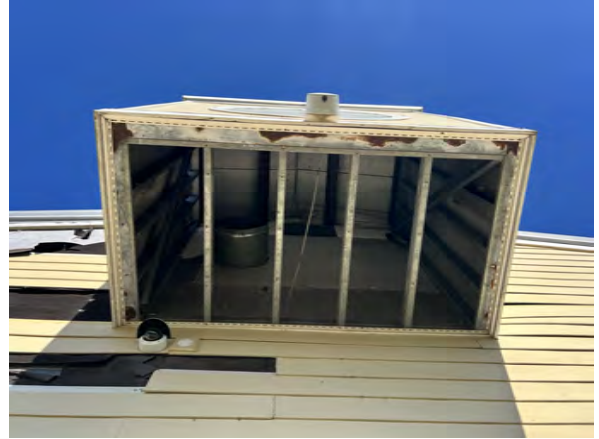
Figure 8: Underside view of HVAC ventilation structure.
