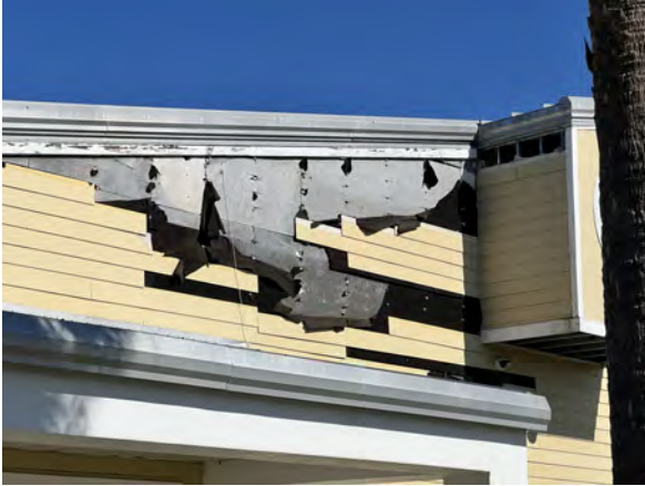
Figure 7: Gable end damaged siding near HVAC ventilation.
