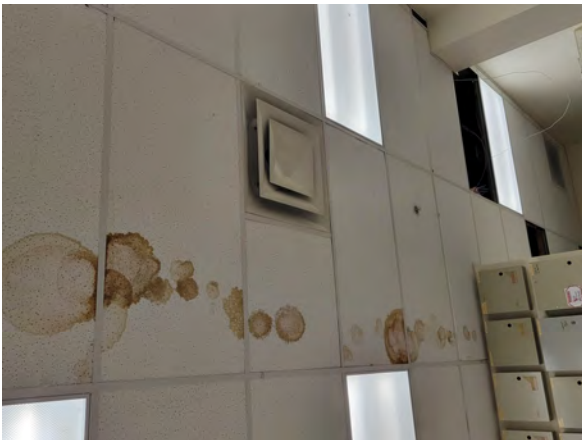
Figure 26: Water infiltration stains on acoustic ceiling tiles.
