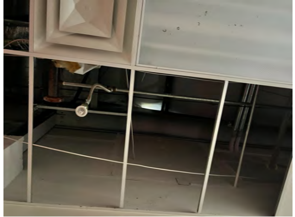
Figure 29: Daylight visible through missing tiles.
