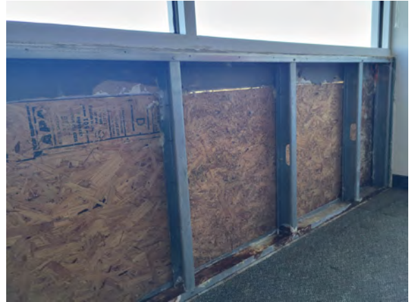
Figure 21: Drywall as sheathing visible with daylight through the cracks.
