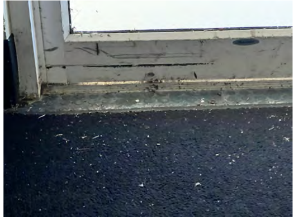
Figure 25: Daylight visible between door and threshold.
