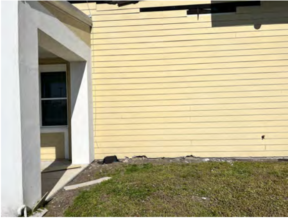
Figure 10: Damage to lower portion of wall siding.
