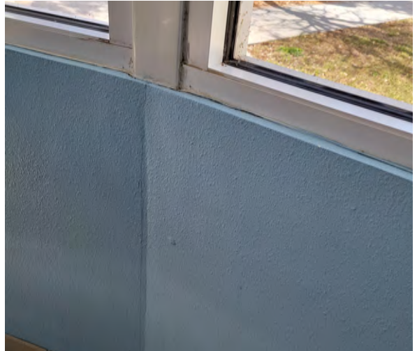
Figure 17: Cracks in drywall and separation of window and wall.
