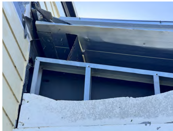
Figure 6: Closer view of exposed framing members.
