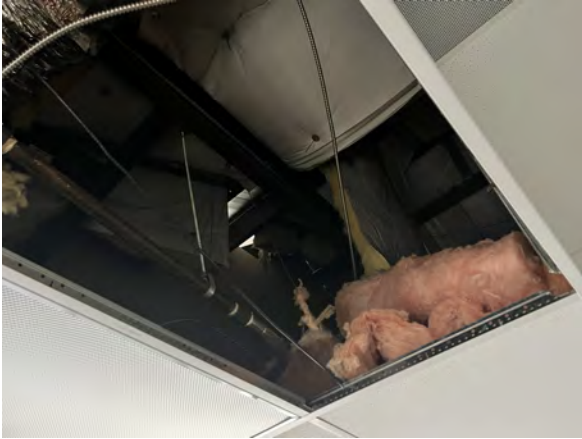
Figure 28: Missing acoustic tiles in ceiling.
