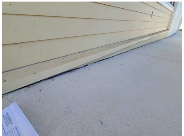
Figure 13: Minor separation of the slab on grade from the building.
