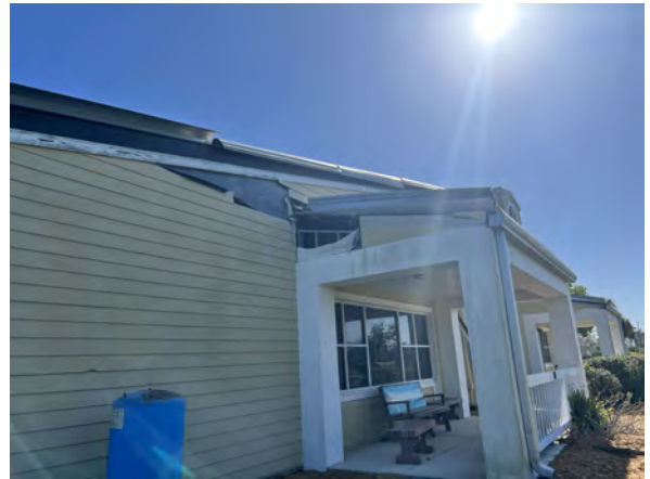
Figure 5: Missing siding with framing elements exposed at side entryway.
