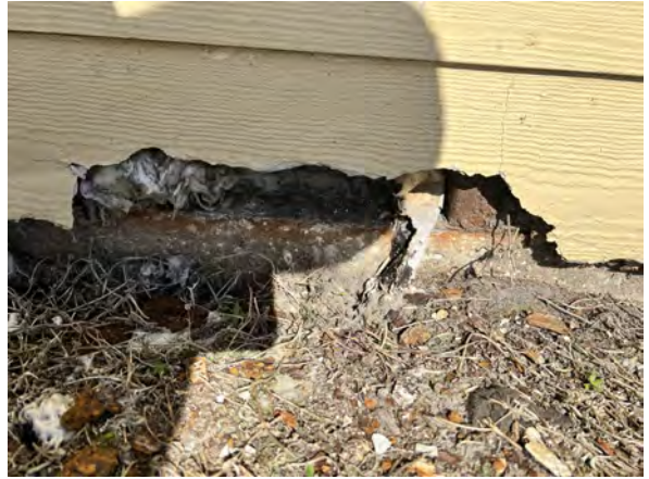
Figure 11: Extent of hole in siding, with insulation and metal stud visible.
