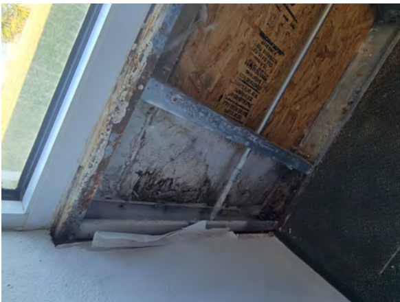
Figure 22: Condition of wall studs and sheathing at corner of wall.
