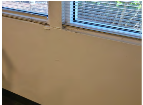
Figure 19: Close view of cracking at window sill.
