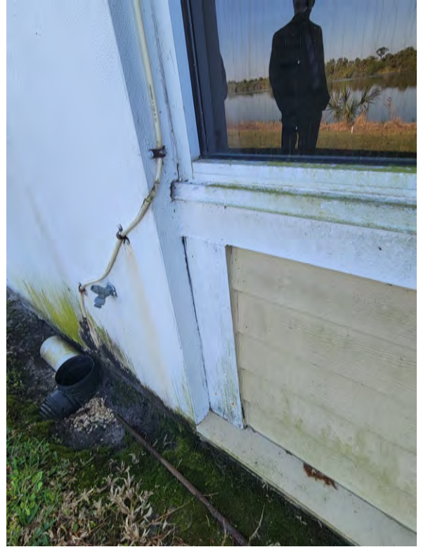
Figure 15: Minor separation of the slab on grade from the building.
