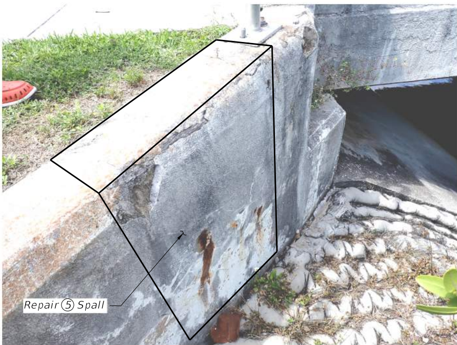
Wingwall Spall (Southeast Wingwall shown)
