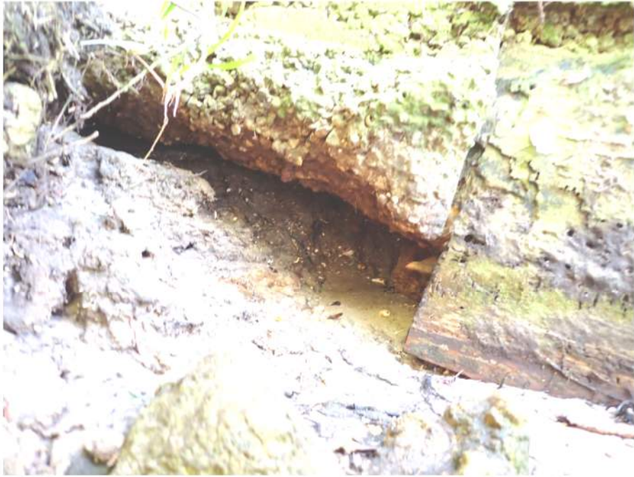
Erosion Along Slope Protection (North Edge of East Slope Protection shown)
