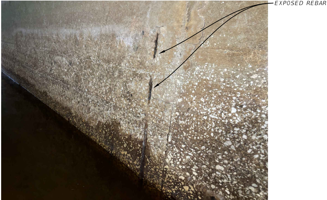
PHOTO 14 - CELL 1, WALL 2, LEFT WIDENING JOINT
