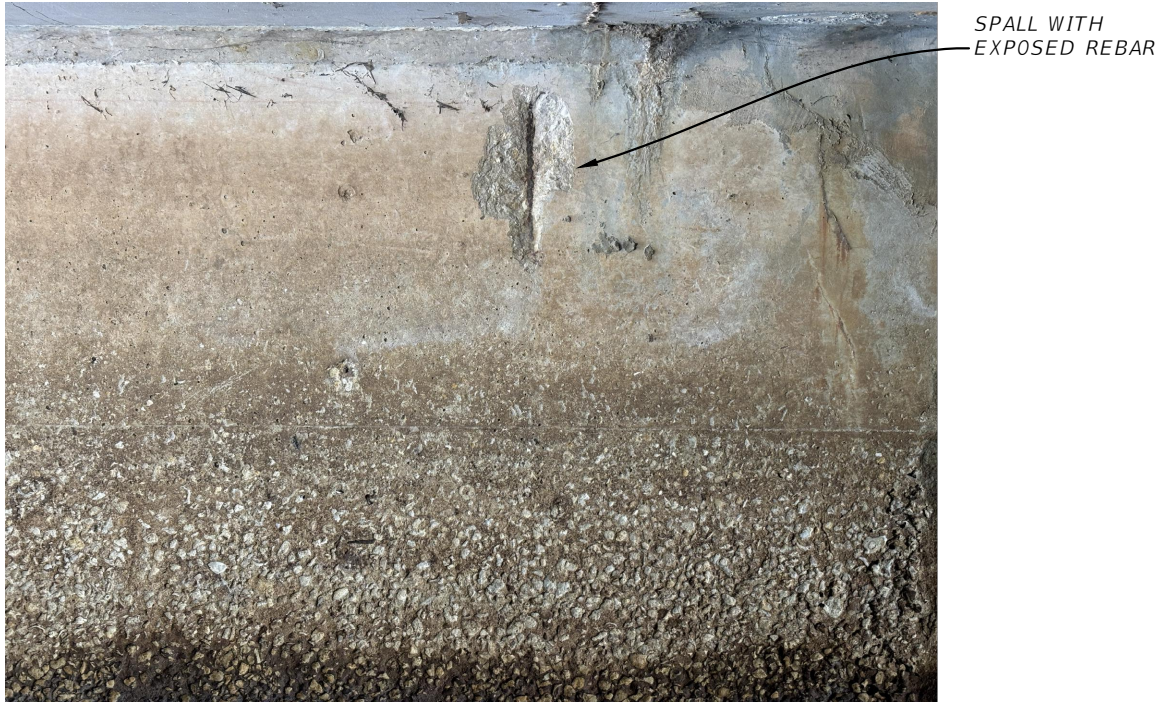
PHOTO 13 - WALL 1, RIGHT WIDENING JOINT
