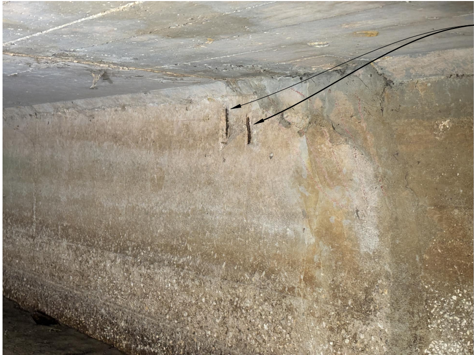
PHOTO 17 - WALL 3, LEFT WIDENING JOINT
