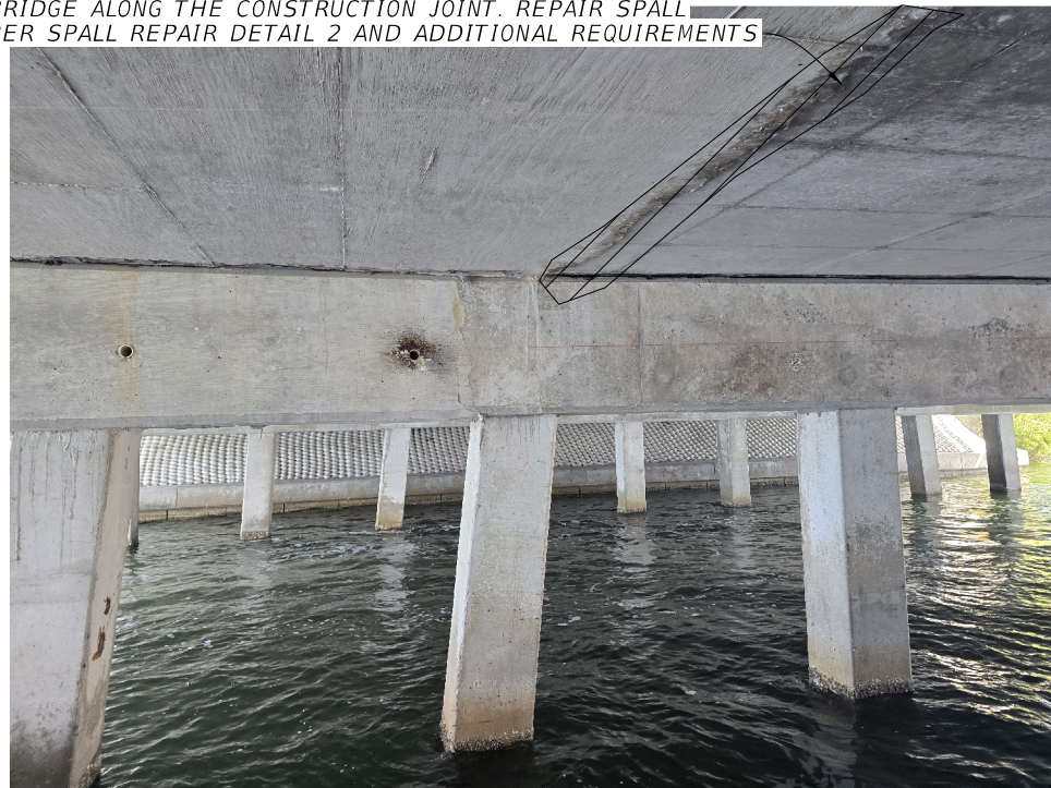
PHOTO 3 - EAST SPALL ALONG CONSTRUCTION JOINT
