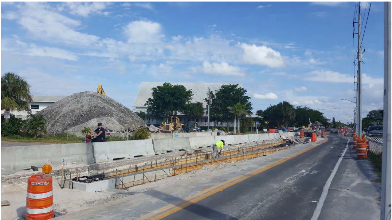
Figure 9: Roadway reconstruction will be necessary to improve walking, biking and driving conditions for all roadway users in Charlotte County. Estero Boulevard in Fort Myers Beach is pictured above.
