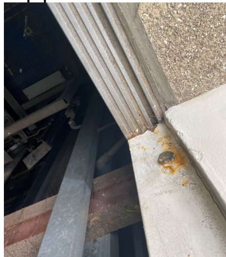
Car 2: Rust on door jambs
