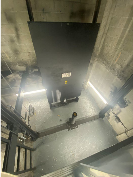
Car 2: Elevator Pit
