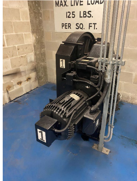
Car 1: Hoist Machine
