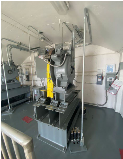
Car 2: Hoist Machine
