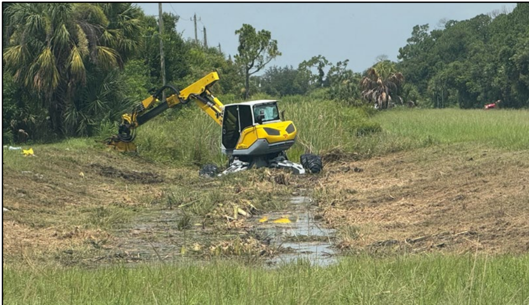
Figure 22: Vegetation maintenance operation in local drainage way, which is fully impacted by cattail growth.
