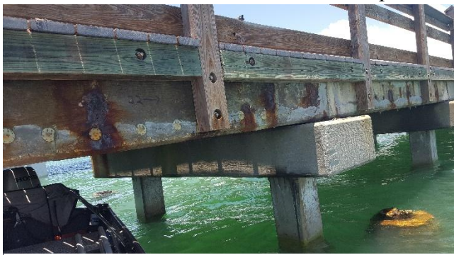
Condition of concrete elements on Anger Pier in 2019
