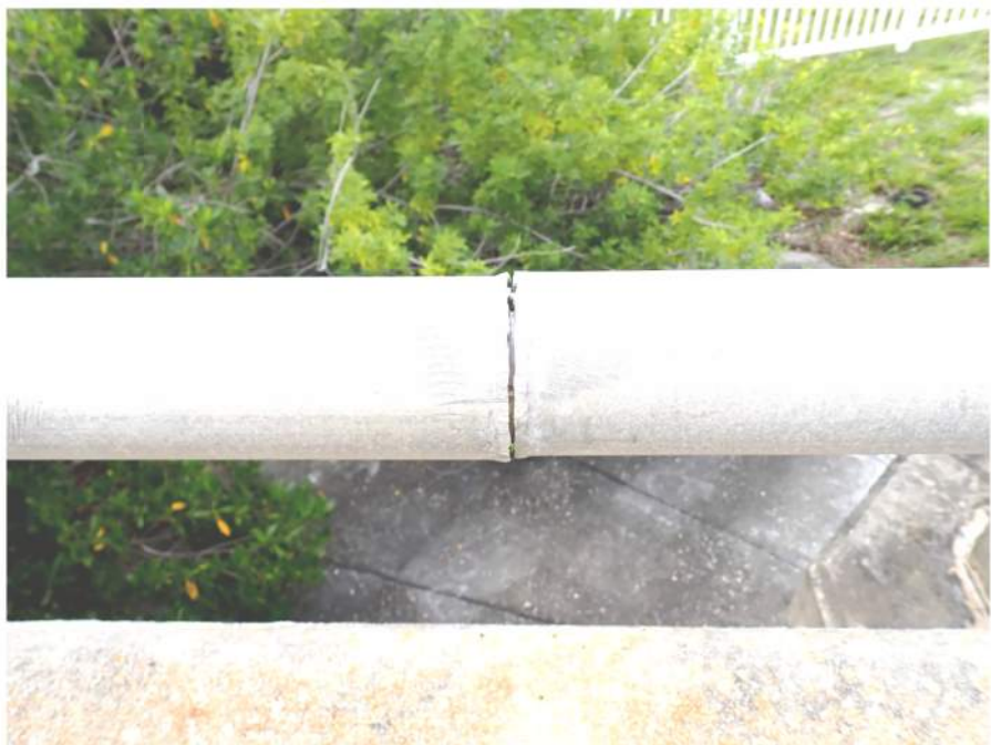
Broken Pedestrian Handrail (Northwest shown, others similar)
